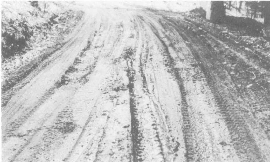
Figure B-2. High severity example of improper cross section.
