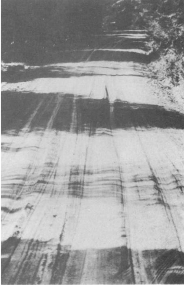
Figure B-12. Low severity example of ruts.
